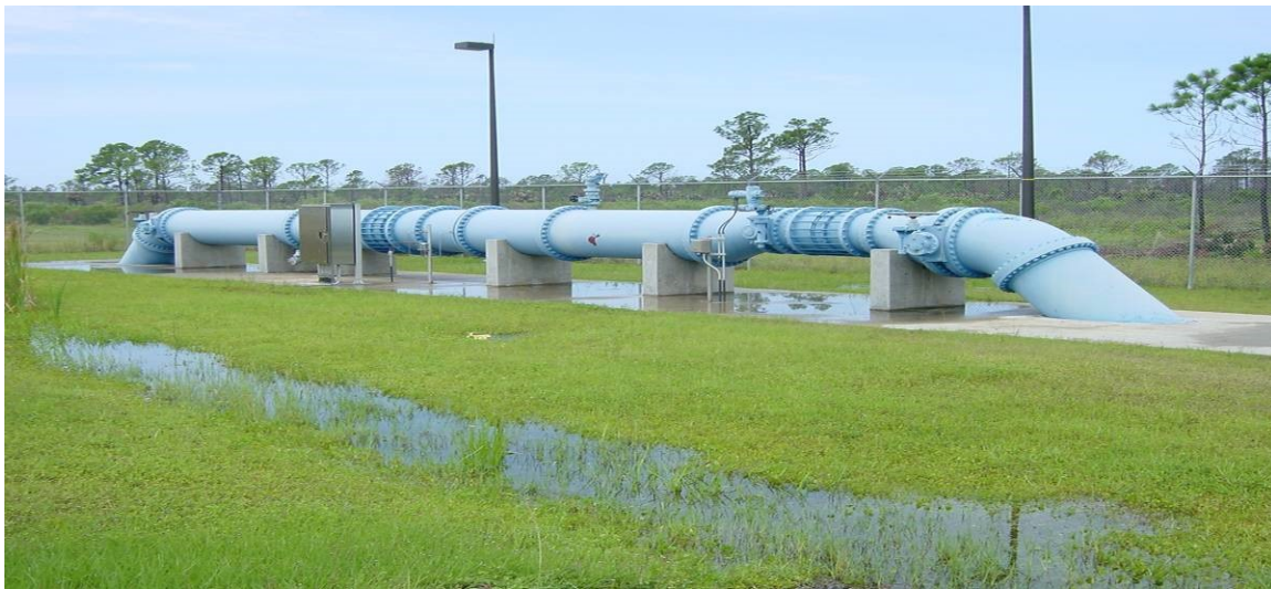
Photo 6. Above-ground meter assemble pipe.
